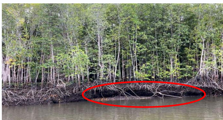
Figure 5: Erosion areas (red circles) were observed in the Tanjung Rhu mangrove forest, with exposed mangrove roots indicating sediment loss and reduced substrate stability, thereby increasing the potential risk of tree collapse.
